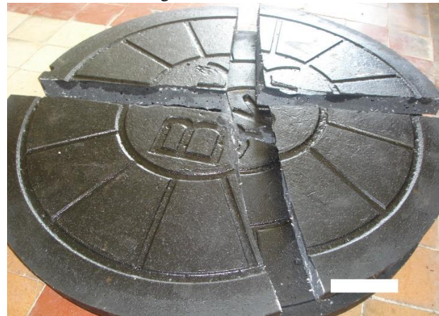
Fig. 7. The nature of the destruction of the hatch cover
