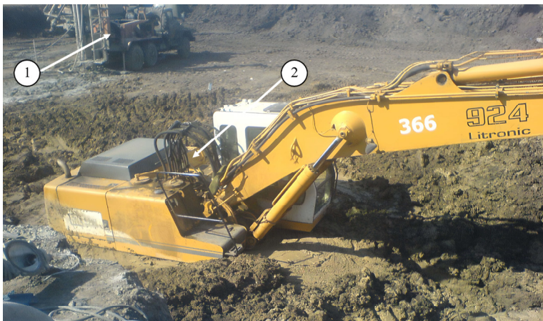
Fig. 6. Arrangement of soil-cement elements under conditions of difficult access: 1 – drilling rig from the proposed BM-811 mechanization assembly (weight 21.75 tons); 2 – excavator R 924 Litronic (weight 25 t)
